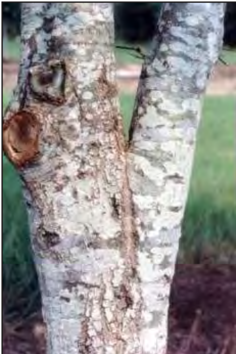
Photo 29. There is included bark in this branch union. The branch bark ridge is not visible because it is included inside the union. The union with included bark is shaped like the letter V.
